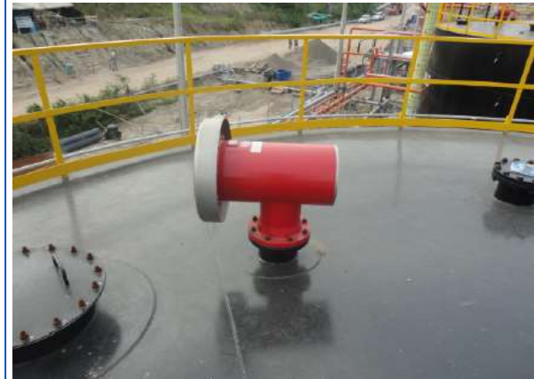
Installed incorrectly (vertical)
